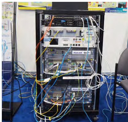
RCP rack for the demonstrations
